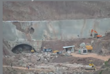
Figure 3: Cavity being tackled at tunnel T-42/43
