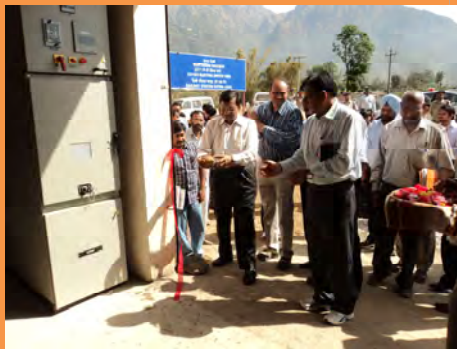
# 4 Sh. Kul Bhushan, Member Electrical and Member Engineering (additional Charge) energised 5MVA, 33/11kV Railway Grid at Katra on 08.04.2013.
