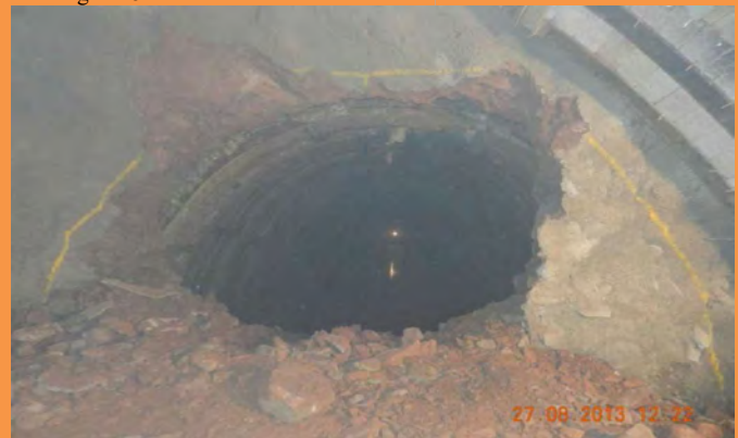
# 6 Break through was achieved at Tunnel No. T42 in Sangaldan area on 27.08.2013. This breakthrough was at the junction of 2 track tunnel with single track tunnel. The total length of tunnel is 2732 m. With this, KRCL has achieved breakthrough in 8 nos of tunnels out of 14 nos.
